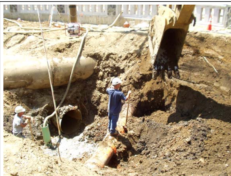
Installation of sewer casing under DELDOT's Newport Road Bridge and existing storm and gas utilities
