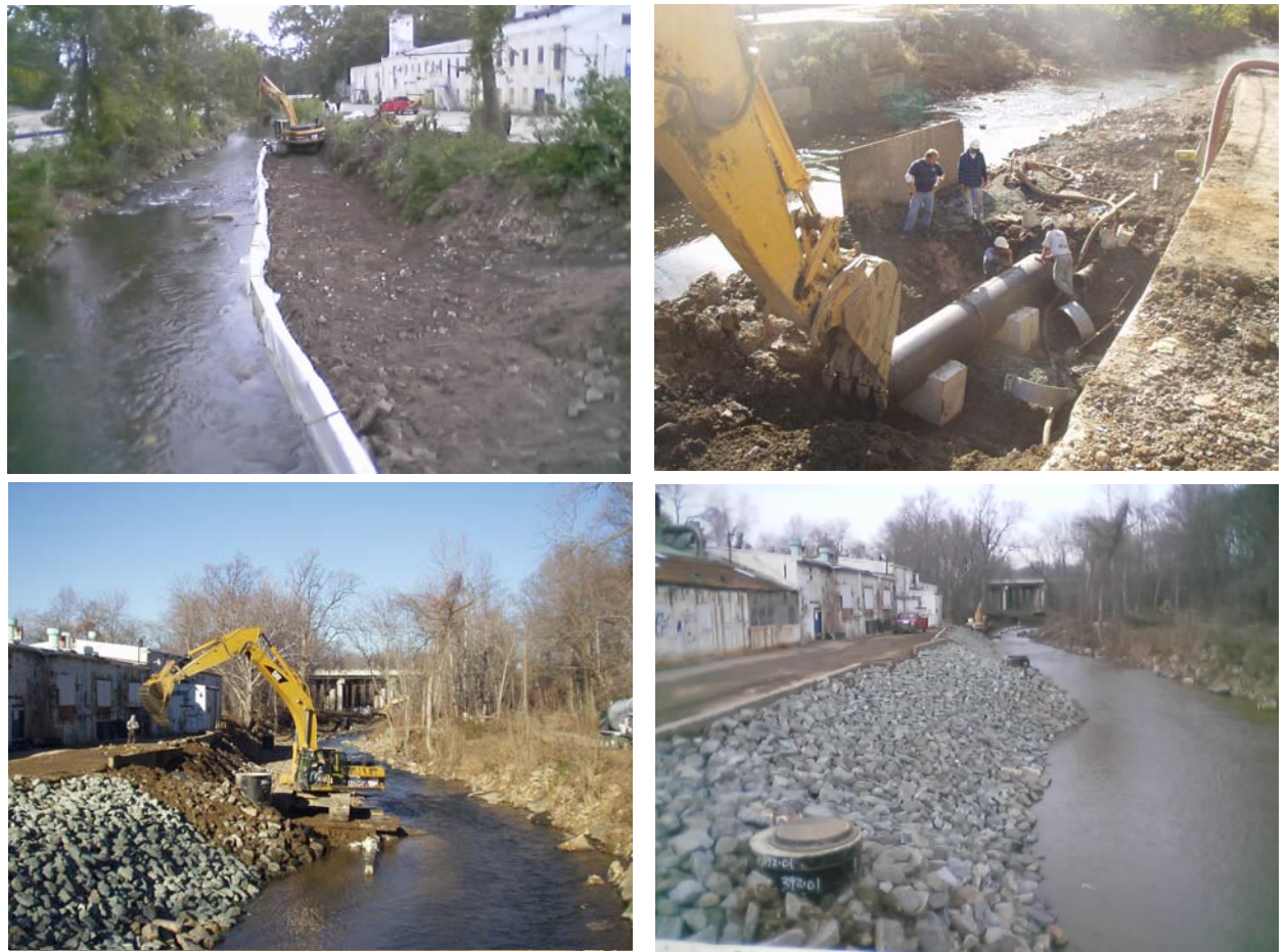
Steps used to replace sewer in the Red Clay Creek (from upper left). 1) Diversion of the stream and creation of a work zone using concrete barriers. 2) Installation of the new pipe with concrete anchors. 3) Removal of the diversion barrier and installation of permanent stone bank. 4) Completed work zone.
