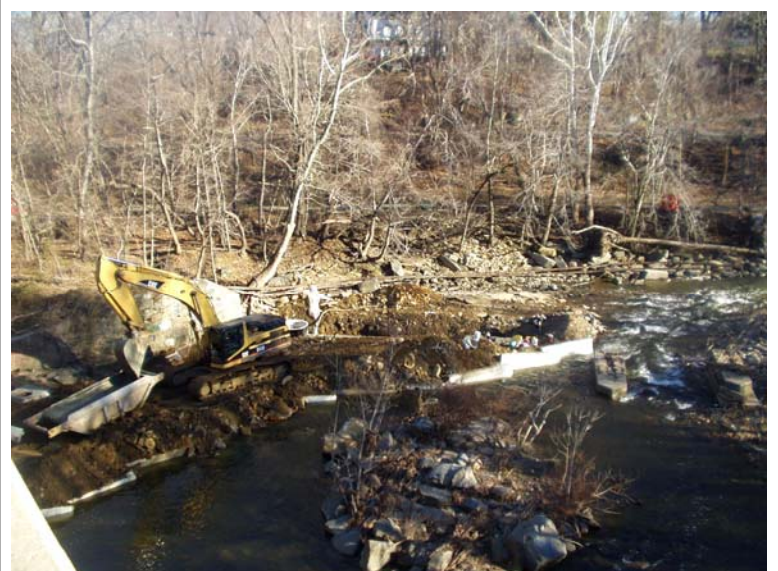
Installation of new sewer across the Red Clay Creek looking down from Kirkwood Highway.
